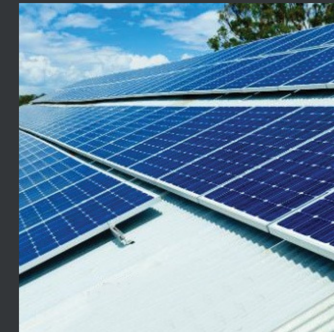
PHOTOVOLTAIC SYSTEM FOR EACH APARTMENT
